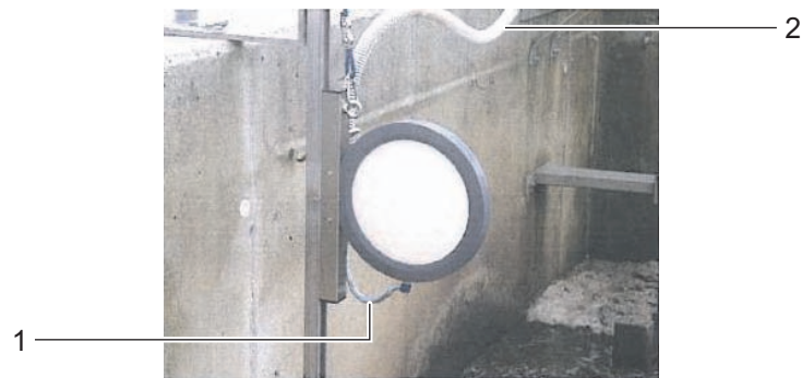
Fig. 5-24: Sample filtration device (installed)
