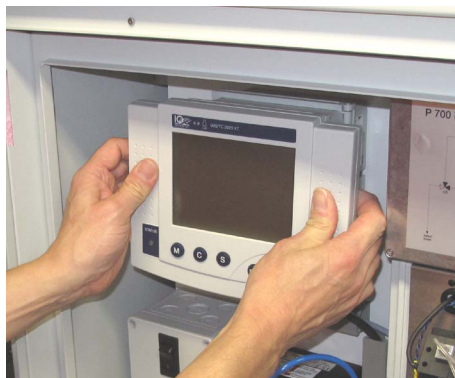
Fig. 4-3: IQ SENSORNET terminal
