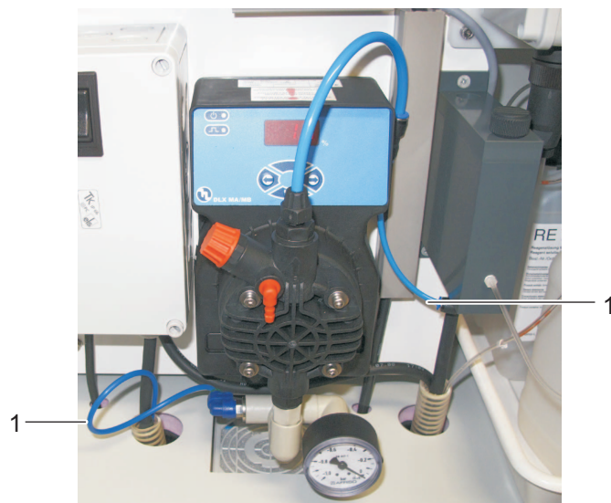
Fig. 5-23: Filtration pump with suction tube
